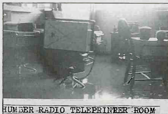
What was left of the teletype room at GKZ once the water receded.
